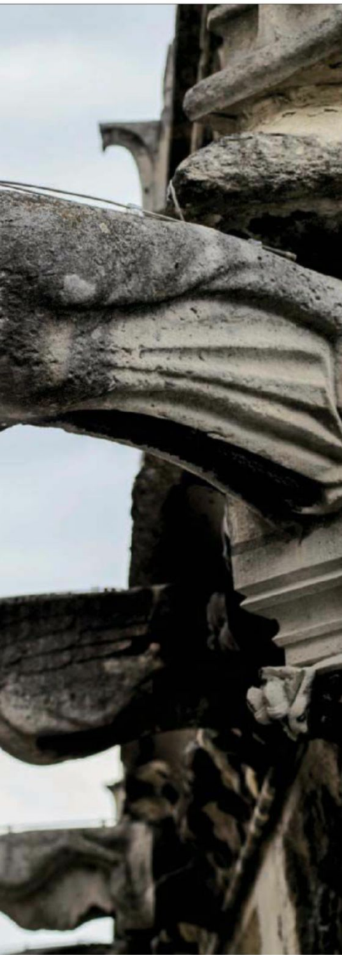
Many of Notre Dame's gargoyles, which act as rain spouts, have corroded and been replaced with PVC tubes
