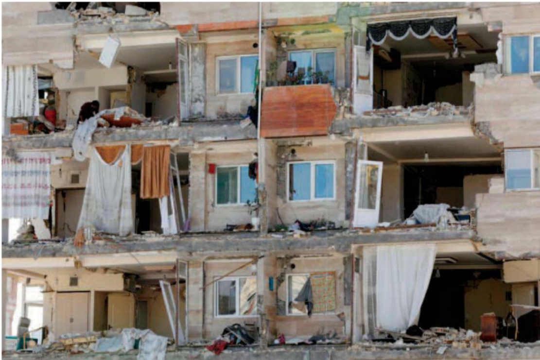
SHORN People search through the debris of their homes on Nov. 13 in the city of Sarpol-e Zahab in Kermanshah province, Iran, a day after a powerful 7.3-magnitude earthquake hit the border area between Iran and Iraq. At least 530 people were killed and nearly 8,000 injured in the deadliest quake of the year worldwide. Iran sits on numerous major fault lines and is prone to near daily tremors. Photograph by Abedin Taherkenareh—EPA-EFE/Shutterstock
