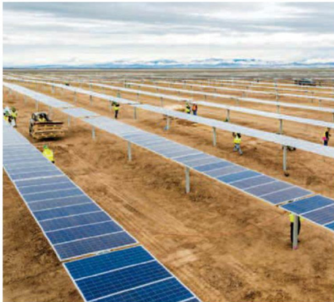
Lit up: Construction crews assemble solar modules for a 55-megawatt power plant in Idaho built by DEPCOM
